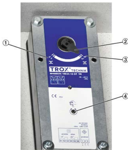
Fig. 39: Open/Close actuator (smoke control damper is open)
